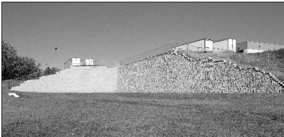
10 meter high wall supporting the truck loading dock area of a commercial development.
