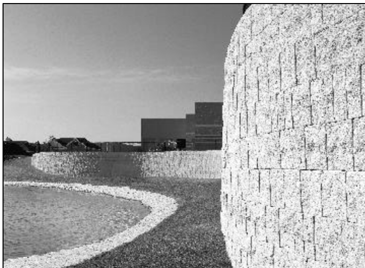
South Carolina commercial development. 4 meter high wall supporting parking and drive areas.
